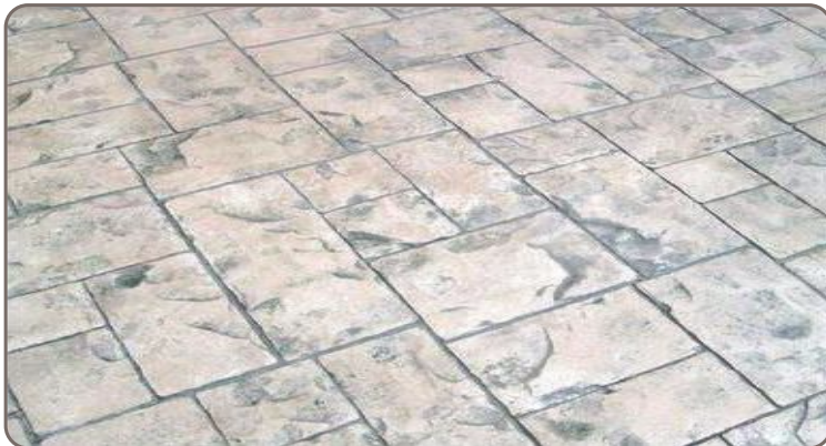
BEFORE: Old, faded, worn stamped concrete.
